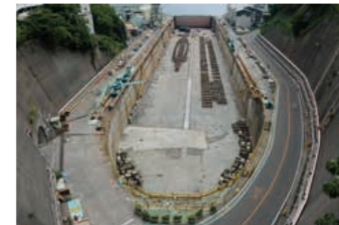
Mitsubishi Heavy Industries Ltd.
