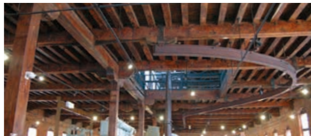
Rail used for transporting materials to the foundry next door still remain. "Nagasaki Yugaku 8" (Nagasaki Bunken-sha)
